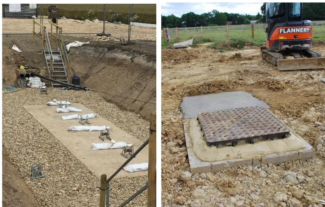
Figure 1.13 a: A typical jointing pit under construction. b. typical link box cover once backfill (image courtesy of RWE Renewables)
